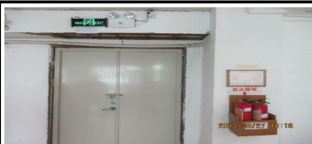
Emergency exit and emergency light
